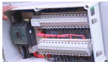
Gambar 8. PVBx (Photovoltaic Combiner Box) (Sumber: Foto hasil penelitian)
