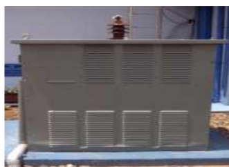
Gambar 1.2 Neutral Grounding Resistance
