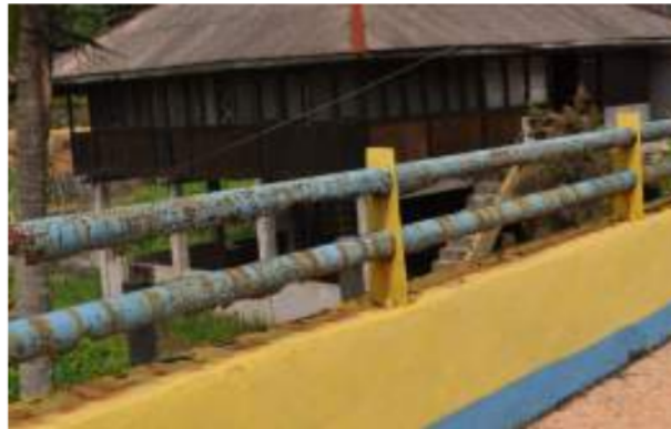
Figure 7: The bridge grip is rusty.
