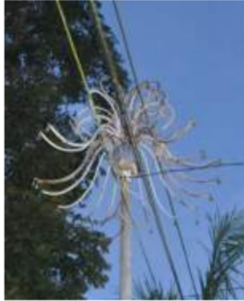
Figure 10: Dangerous Street Lights.
