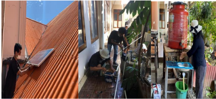
FIGURE 5. The installation and implementation of solar water pump system in Bunaken island
