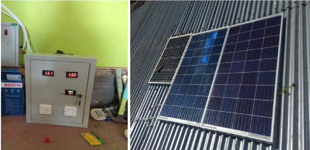
Gambar 8. Produk Alat Monitoring Panel Surya
