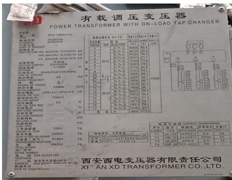
Gambar 1 Name Plate Trafo
