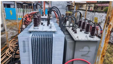
Gambar 2 Transformator PLTD Laiwui
