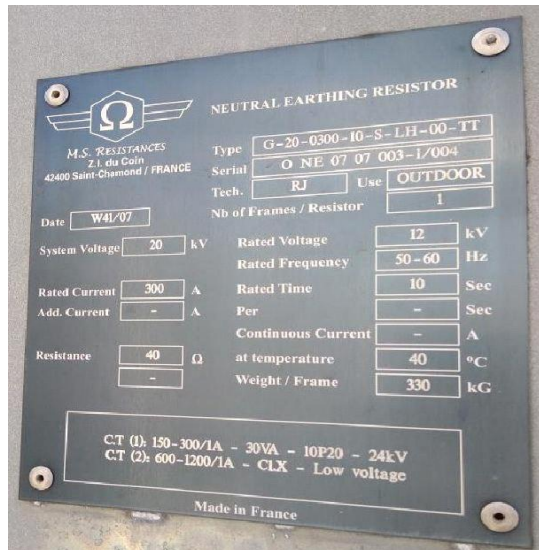
Gambar 2. Name Plate NGR (Netral Ground Resistor)
